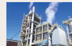
Woody Biomass Power Generation Facilities, Ono City, Fukui Prefecture (Equipment installation work)
